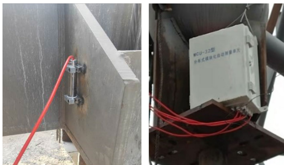
(a) Vibrating wire strain gauge
