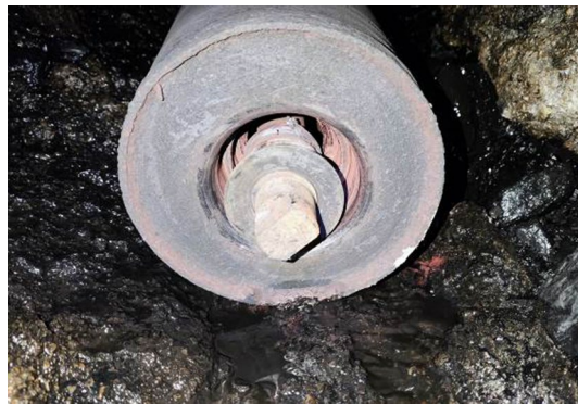
Figure 9. Malfunction roller of rack 58.
