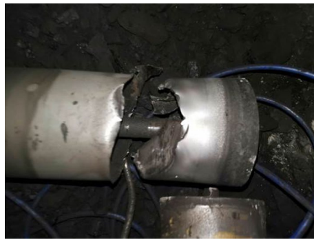
Figure 13. Malfunction roller of rack 24.
