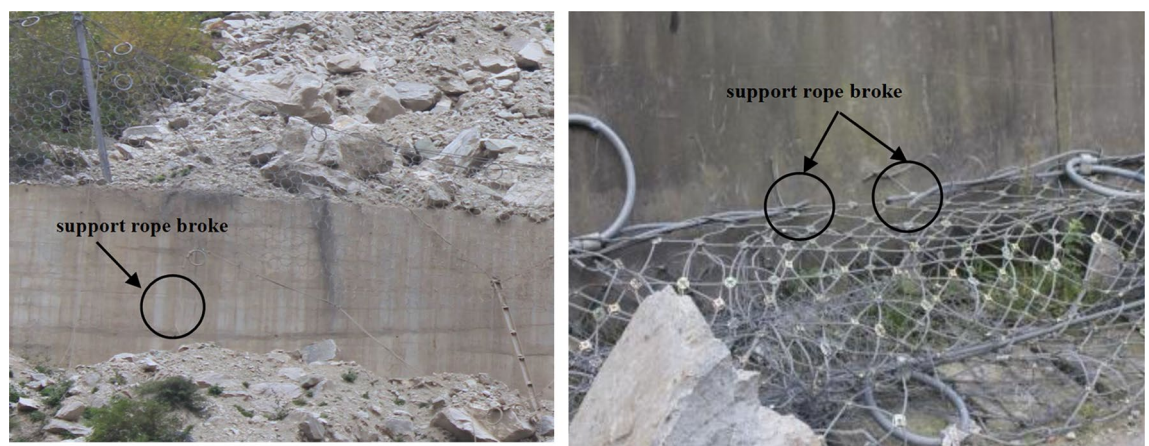
Figure 2. Broken support rope.
